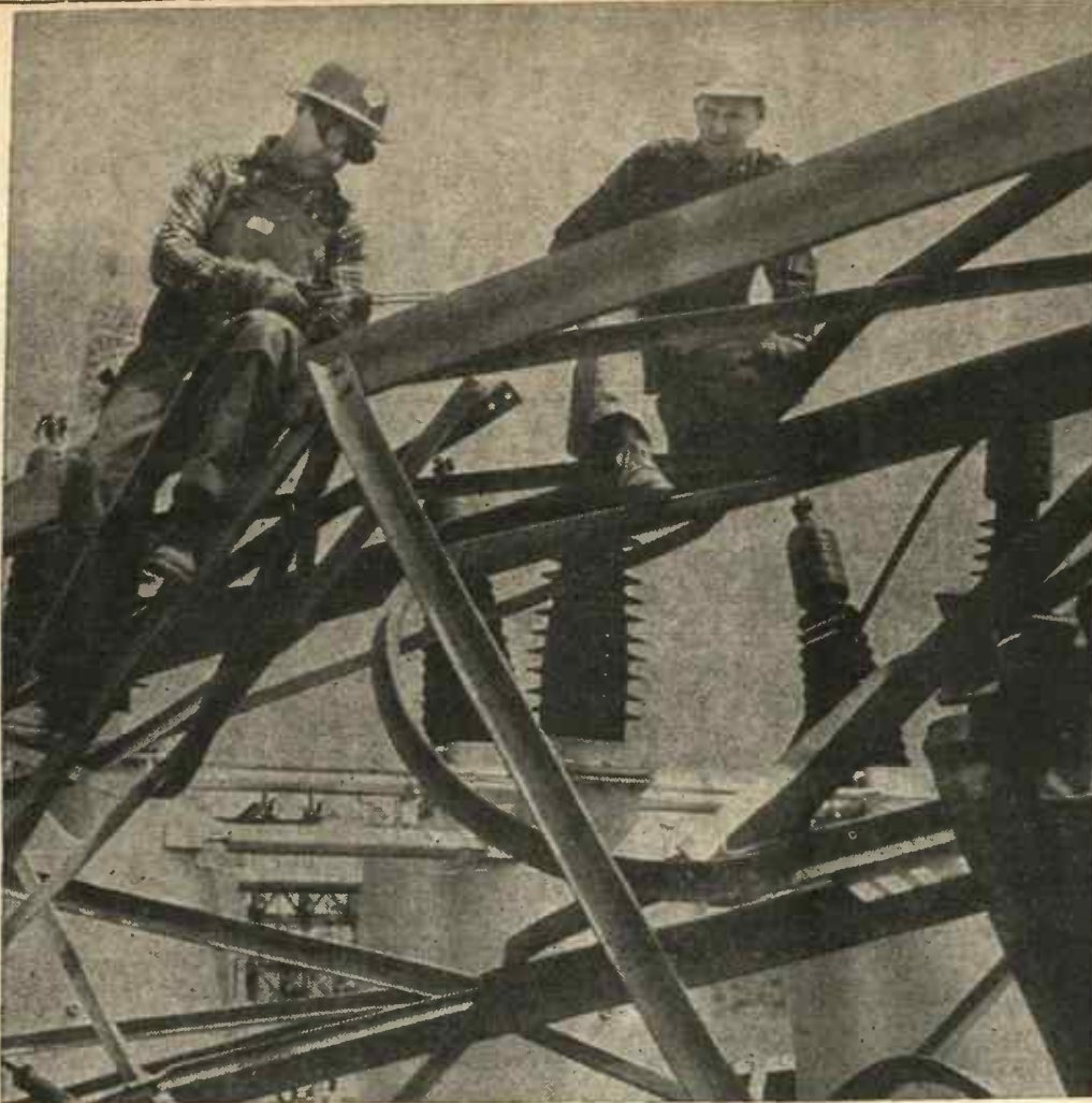
STEEL STRUCTURES DISMANTLED —TVA crews are dismantling twisted steel structures leveled by a tornado March 4 at Pickwick Dam switchyard in southwest Tennessee. The switchyard feeds electricity generated at the dam into the transmission system. Estimates of total damage are not complete, TVA said, but changes in the system since the Pickwick switchyard was originally installed will make it possible to restore the transmission connections for much less than the original cost.
